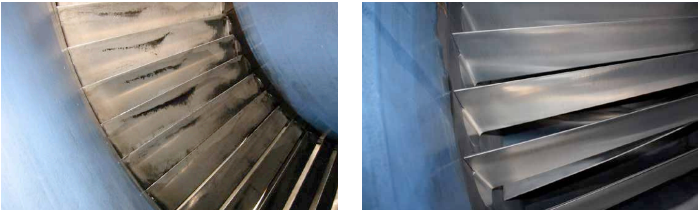
Figure 1: Inlet guide vanes (left) after 1,200 hours of lower-efficiency filtration (Er2), compared with the same inlet guide vanes (right) after 5,000 hours with higher-efficiency filtration (Er5).
